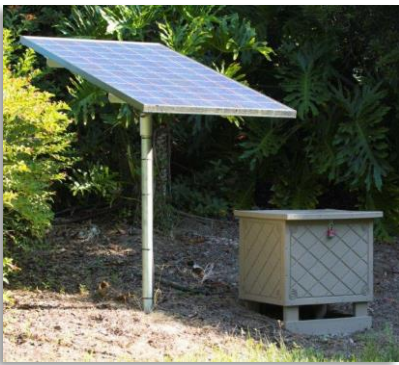
Solar Panel & Cabinet
